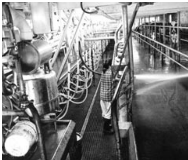
This operation modernized by adding a pit parlor, which improved labor efficiency and milker safety.
